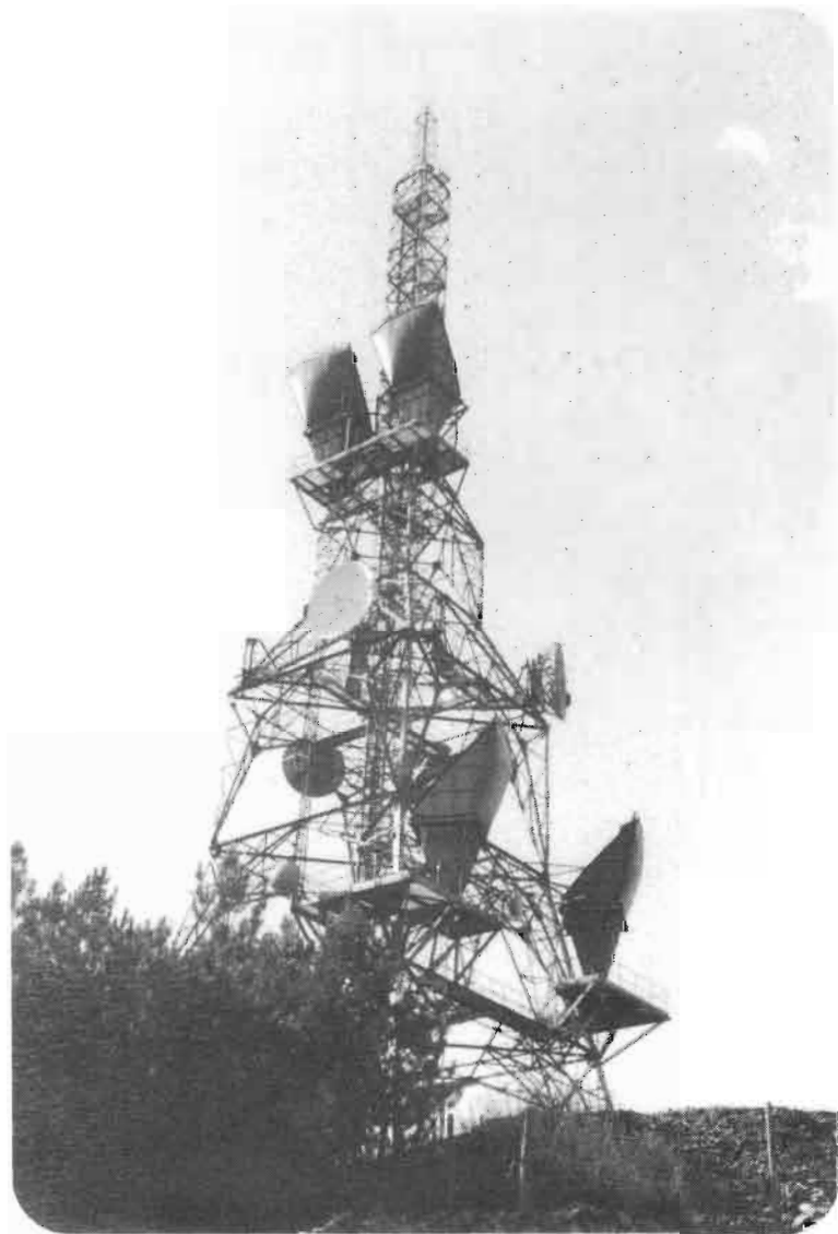
FIGURE 3. The tower at the Riddings Hill communications station (Photograph by Tom Straiton)
